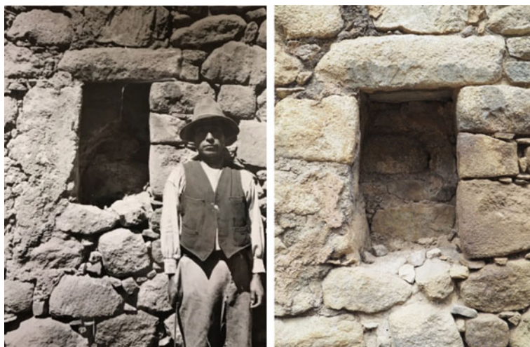
Fig. 10.16 Comparative analysis of the plaster in the niche of the structure 08 (plaza 1). Left: 1941 photograph by Paul Fejos; Right: 2017 photograph by Dominika Sieczkowska
